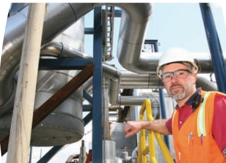
Dave Henden, finish end superintendent at Commencement Bay Operations, checks the steam-oil heater near the kilns.
