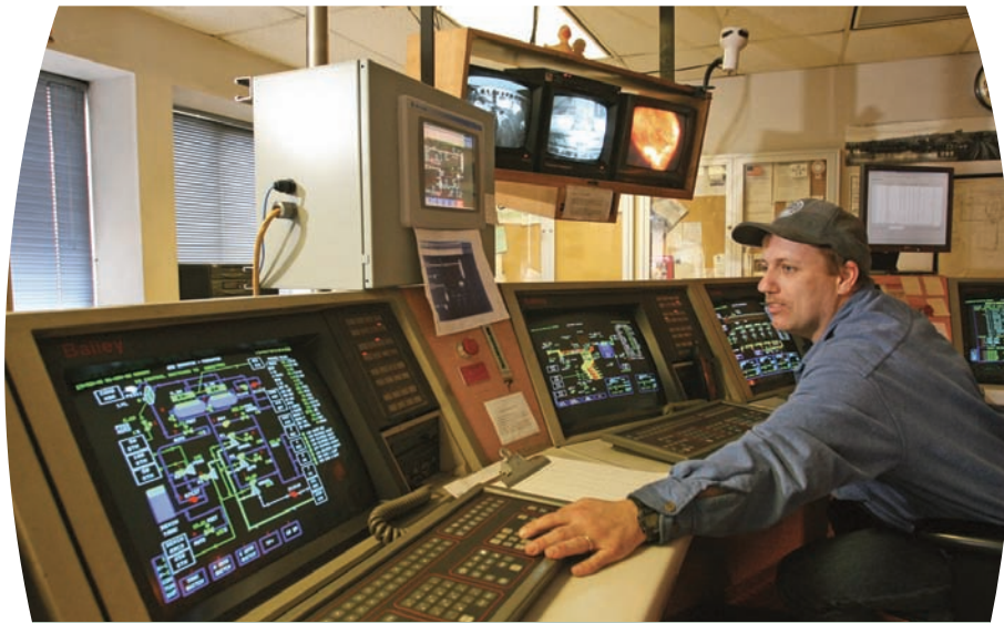
George Skinner, pulp mill operator, handles the number 6 and 7 boilers at Simpson Tacoma Kraft Company. The boilers can produce 460,000 pounds of steam per hour or 46 percent of the total steam output at the mill.
